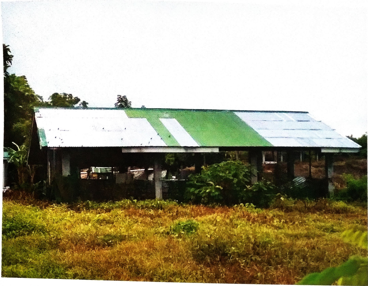
Damaged Duck House
