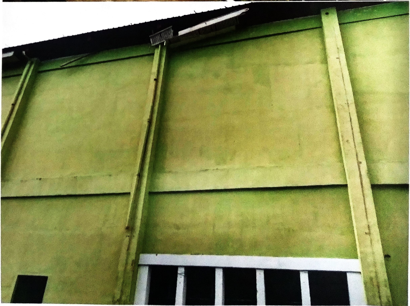
DAMAGED OVERHANG CEILING, FASCIA AND DOWN SPOUT OF PACKING HOUSE DA RFO 5, Pili, Camarines Sur
