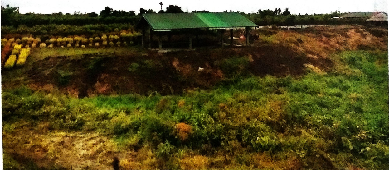
Damaged Roof, flashing and fascia of Palay Sheds at Poultry Production area DA RFO 5 Compound, San Agustin, Pili, Camarines Sur
