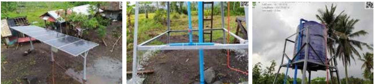
Installed Solar-Powered Irrigation System in Albay
