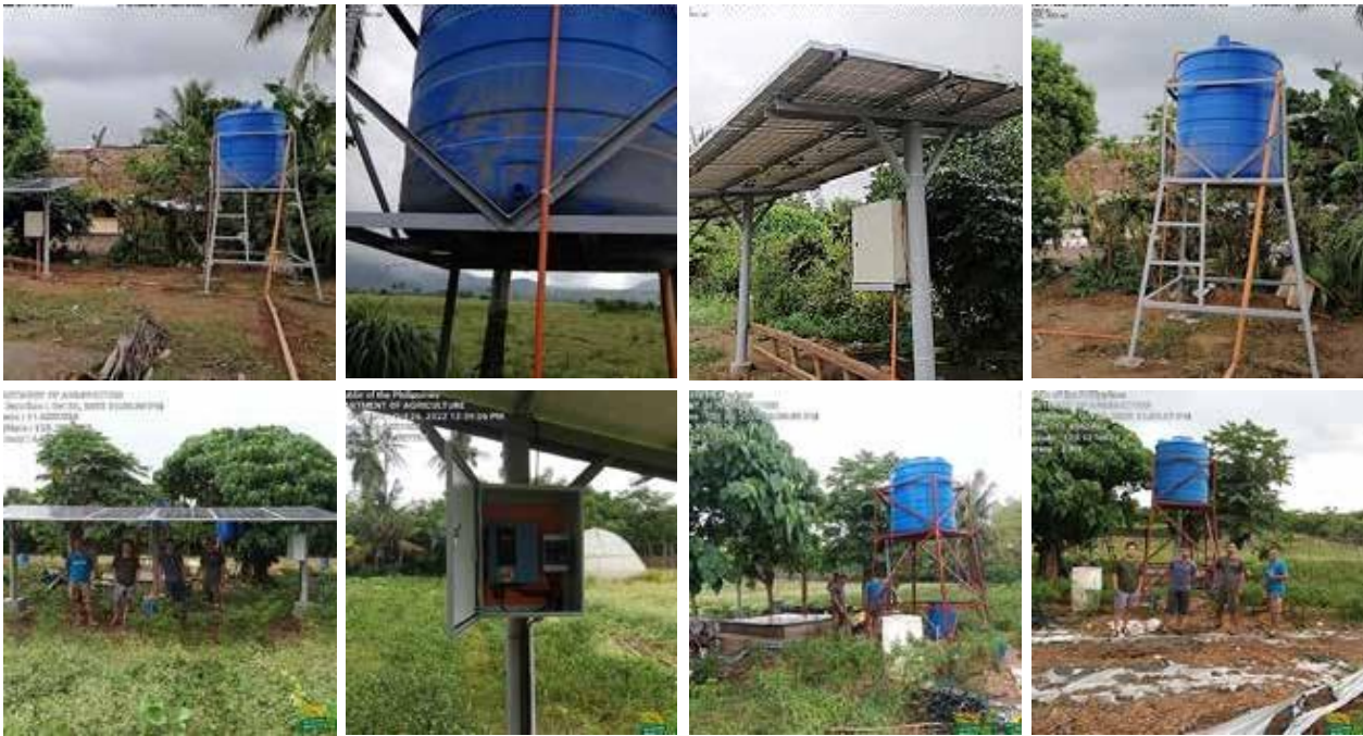
Installed Solar-Powered Irrigation System in Sorsogon
